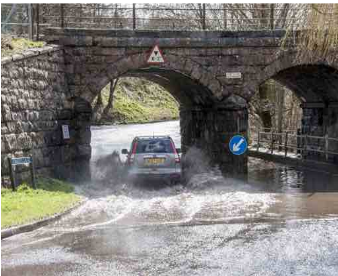
Figure 33 (left) - Railway Bridge on Jobbers Lane affected by river water flooding, March 2016
